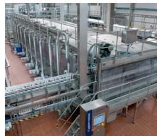
Optimised insulation of the pasteuriser can further reduce heat loss.
